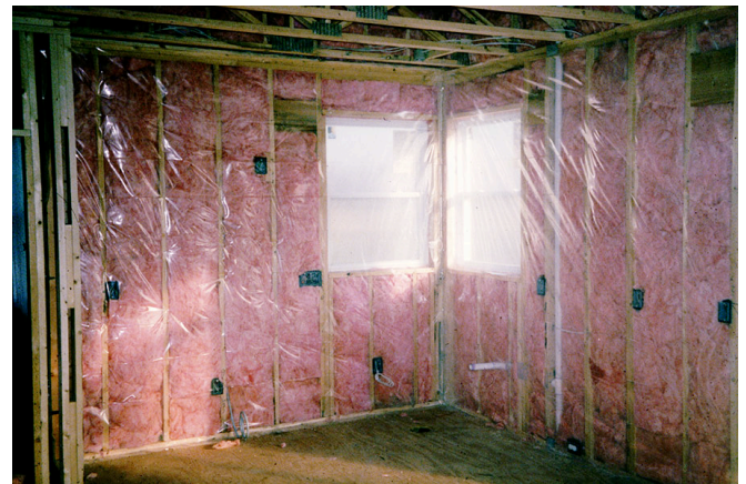
Photograph 3: Interior Polyethylene Vapor Barrier —The sheet polyethylene on the interior is clearly a vapor barrier. In this assembly it is also acting as an air barrier (air control layer).
