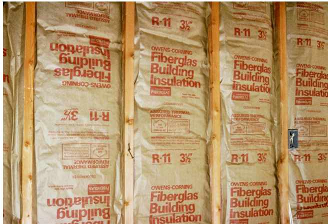
Photograph 4: Kraft Faced Fiberglass Batts —The facing is the vapor control layer. Note that the Kraft facing does not function as an air barrier (air control layer).
