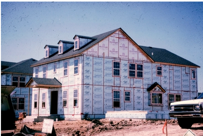
Photograph 2: “Classic” Wood Frame Wall With Foam Sheathing —A wall that we have been building in cold climates for 40 years. The foam sheathing on the exterior is clearly a vapor barrier. The “vapor profile” is that of a “double vapor barrier”. I grew up with this wall in Ontario—2x6 wall with R-5 foam sheathing and a plastic interior air/vapor barrier.
