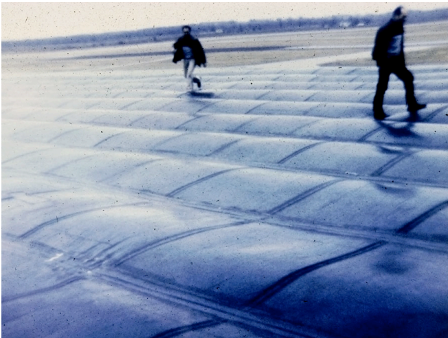
Photograph 1: Missing Air Barrier —With a mechanically attached membrane and no bottom side air barrier the roof membrane “flutters”.
