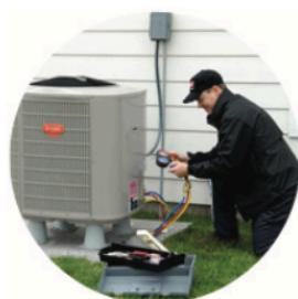
HVAC & Water Heating
